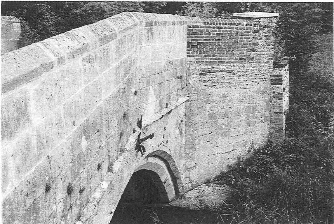
Splay at SE corner
